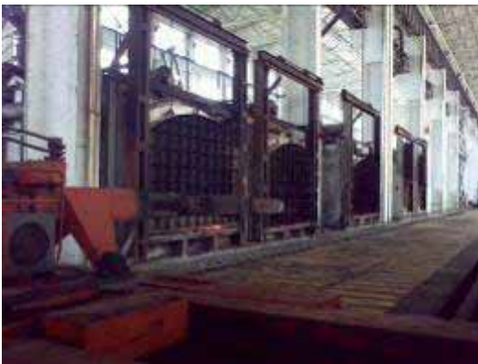
Heating treatment stove
